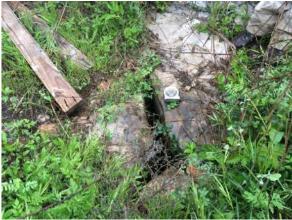
Feature F-6 – solution cavity located along the southern limits of the TxDOT right-of-way south of US290
