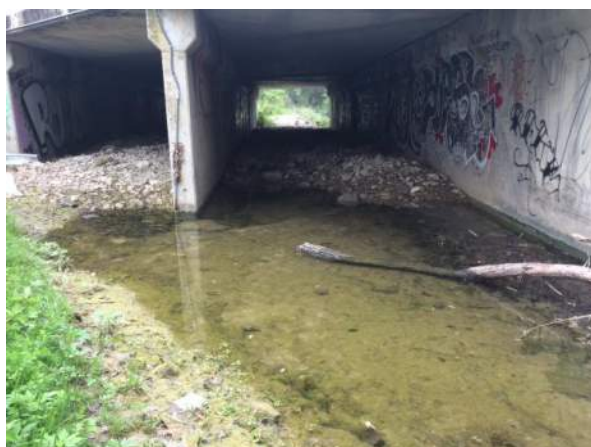
Feature F-1. Widely spaced fractures within the Williamson Creek streambed located just upstream of US290
