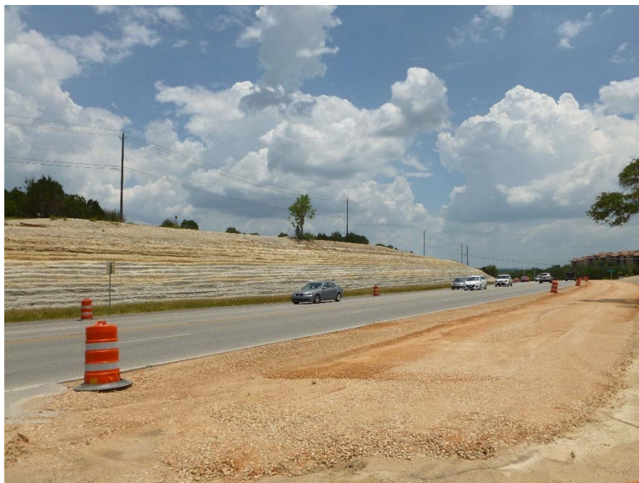
Photograph 9: Roadway cut in front of the Austin Community College Pinnacle Campus; facing northeast.
