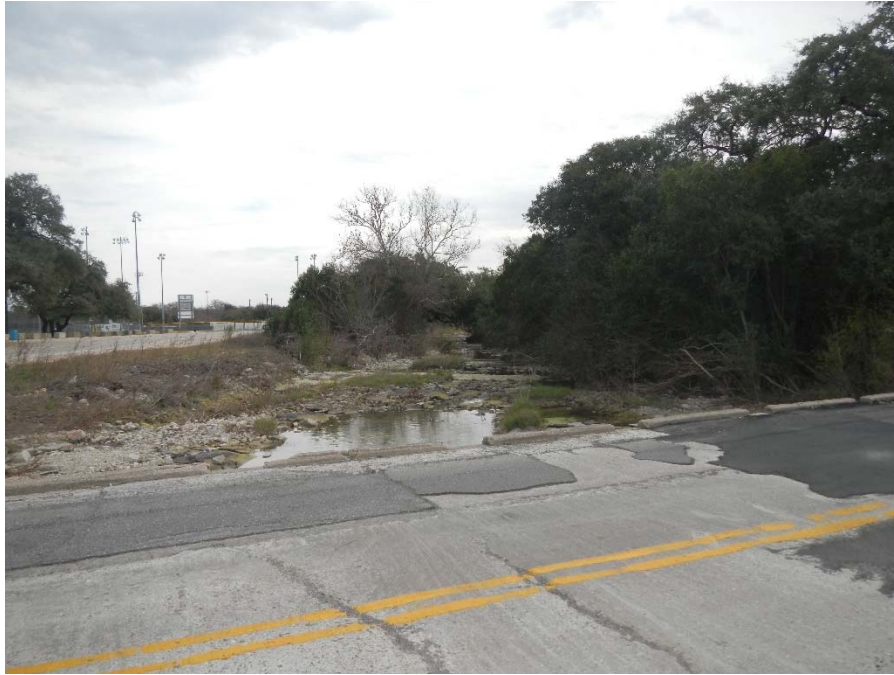
Photograph 19: Low water crossing of Williamson Creek at Joe Tanner Lane; facing southeast.
