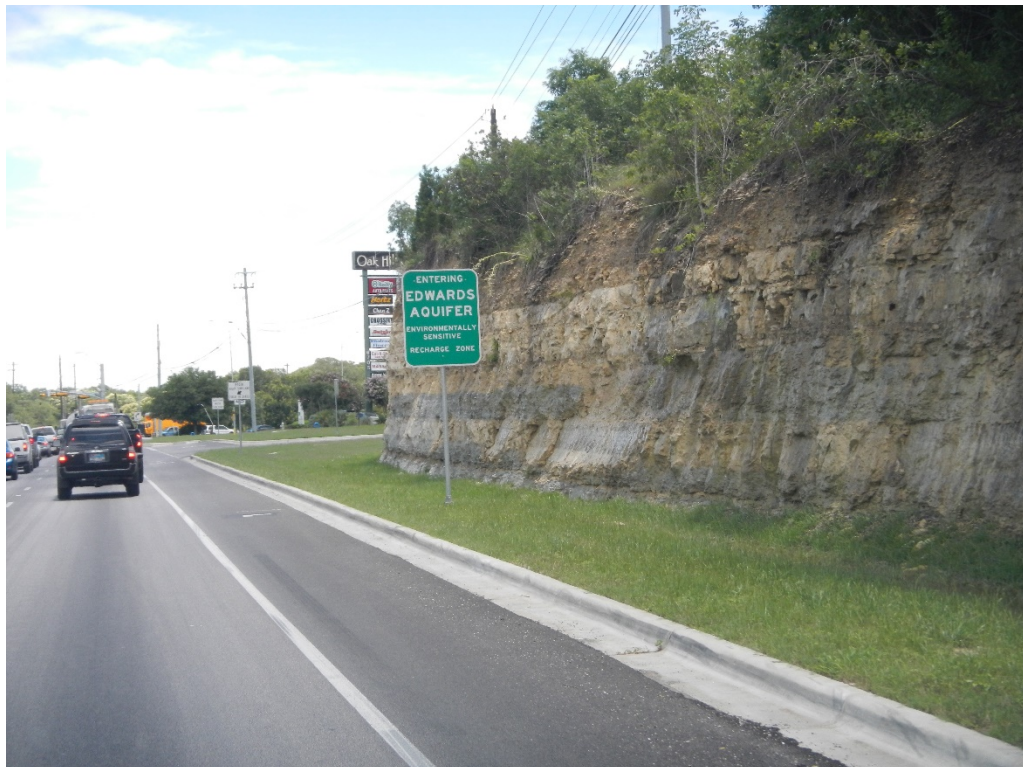
Figure 24. Existing US 290/SH 71 right-of-way west of William Cannon Blvd. Facing east. Note the deep road cut below grade.
