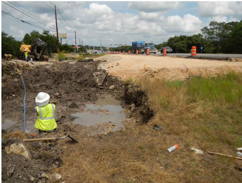
Figure 13. Disturbance from new construction in ROW. Facing northeast.
