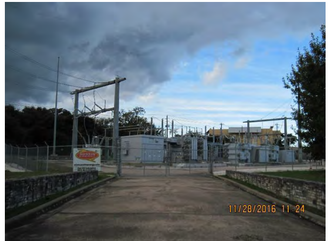
Photo 4: Electrical substation on McCarty Lane just south of project corridor. Photograph taken facing west.
