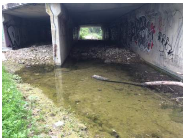
Feature F-1. Widely spaced fractures within the Williamson Creek streambed located just upstream of US290
