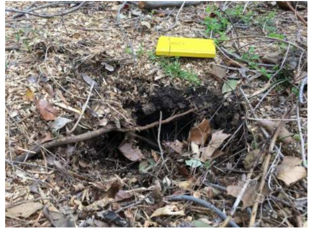
Feature F-7 – Cavity located north of the existing US 290 right-of-way along the transmission line corridor.
