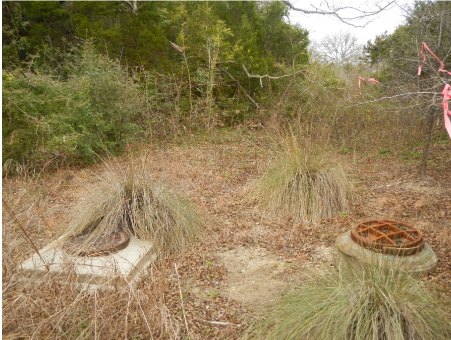
Photograph 17: Utility infrastructure within the Bee Cave detention pond; facing west.
