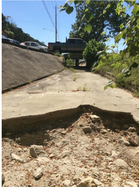
Photograph 33: Unnamed tributary to Williamson Creek (S-7) south of US 290/SH 71; facing east.
