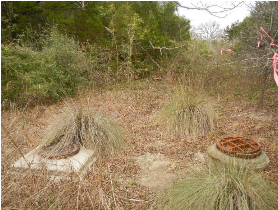
Photograph 24: Utility infrastructure within the Bee Cave detention pond; facing west.
