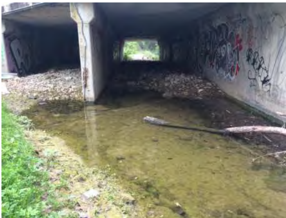
Feature F-1. Widely spaced fractures within the Williamson Creek streambed located just upstream of US 290
