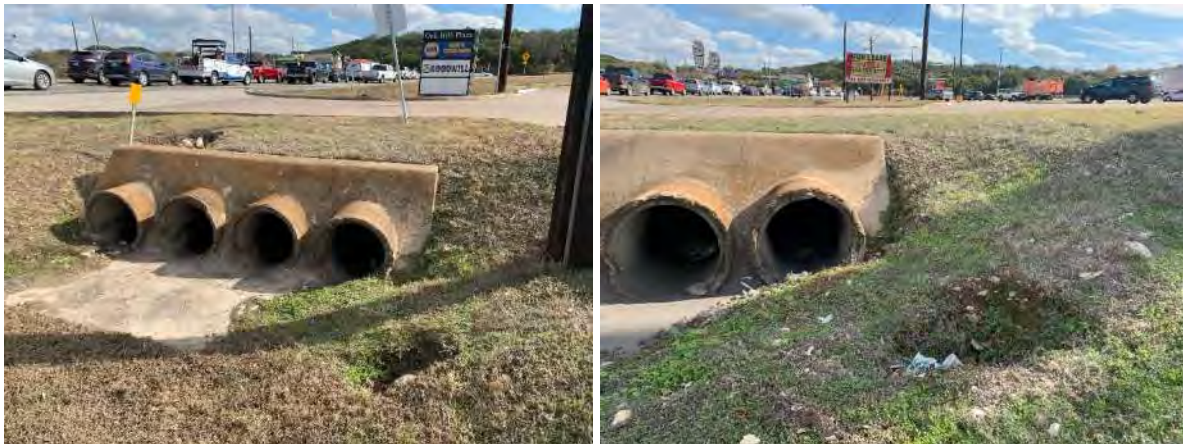
Non-karstic soil slump features identified at two driveways leading to the Oak Hill Plaza shopping center along the south bound lane of SH 71 immediately beyond the split with US 290.
