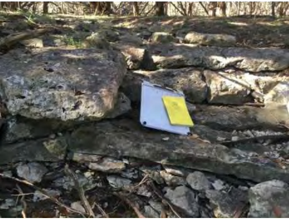
Feature F-9 – Area of fractures located within proposed right-of-way for the detention pond on the southwest side of SH 71.
