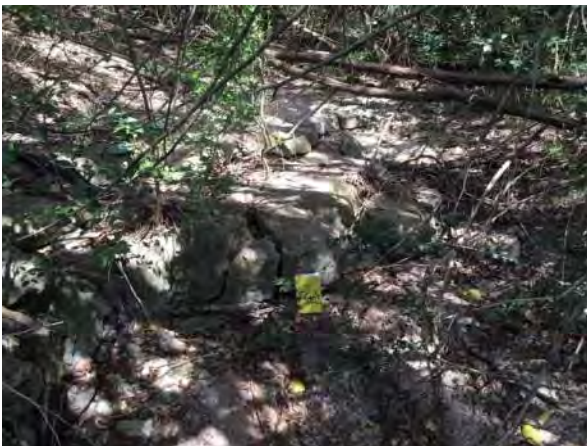
Feature F-8 – Area of fractures located south of the intersection of Old Bee Caves Road and the Bell Hill Country Apartments entrance road. On proposed right-of-way.
