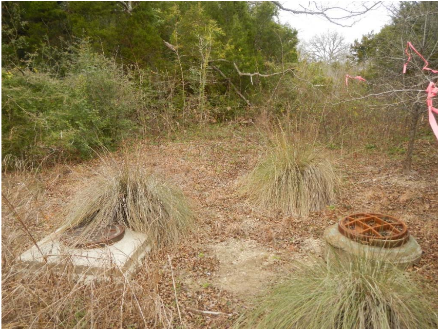
Photograph 14: Utility infrastructure within the Bee Cave detention pond; facing west.
