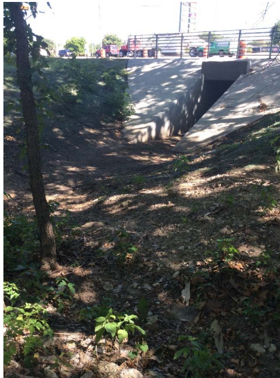
Photograph 31: Unnamed tributary to Williamson Creek (S-8) north of US 290/SH 71; facing south.
