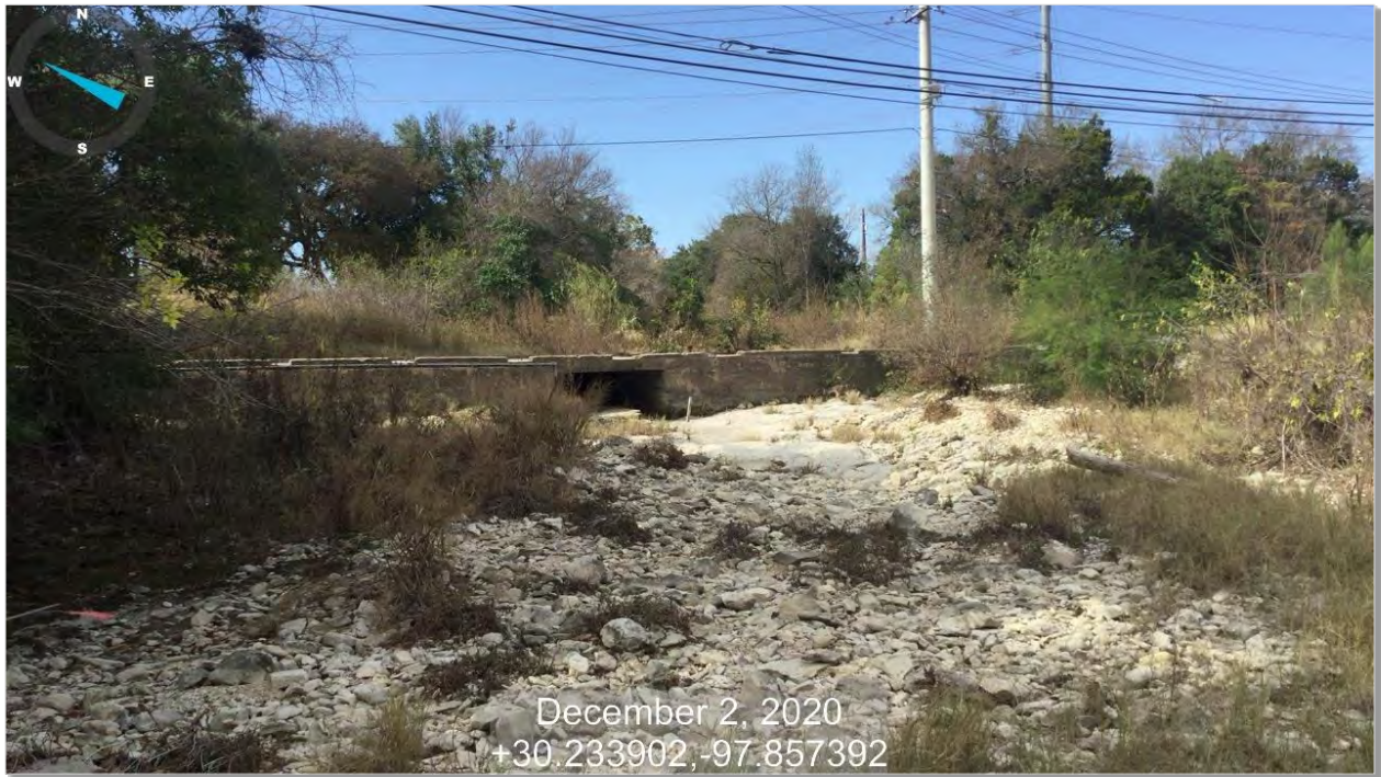
Photo 14: Typical upstream view of stream S-6, an intermittent stream named Williamson Creek at Joe Tanner Lane.
