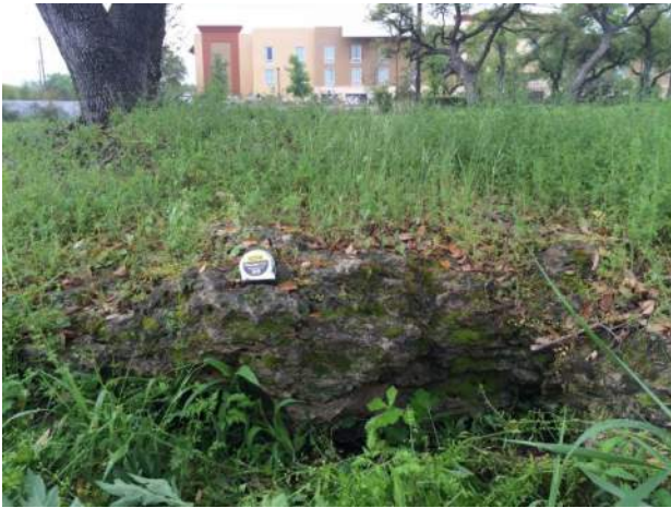
Feature F-4. Zone of fractures located south of US290 along the southern margin of the TxDOT right-of-way
