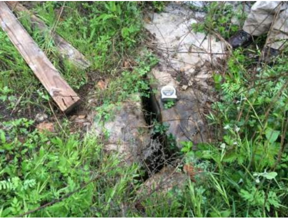
Feature F-6 – solution cavity located along the southern limits of the TxDOT right-of-way south of US290
